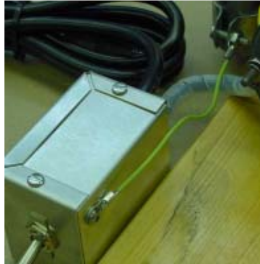
Figure 5 - Motor capacitor bracket ground wire running to switch box ground terminal.
